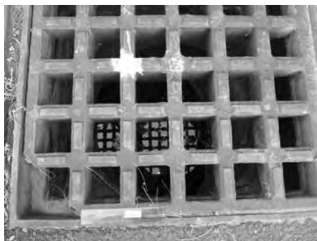
Storm drain, photographs by the authors
